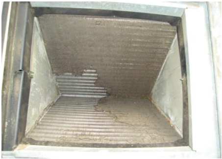
Dirt coating the inside of coil.
